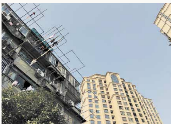
Drying racks fixed on the facades of old mass housing blocks are pervasive due to the absence of balconies or laundry space inside (Jin Zhu)
